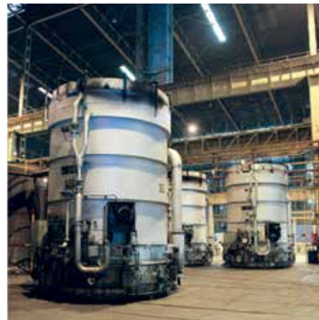
Batch Annealing Furnace
